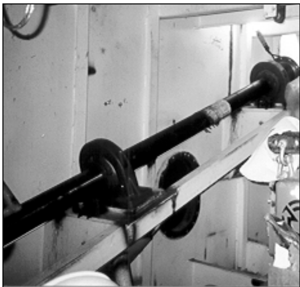
Photo 5 Modified Bearing Supports: Case 3
