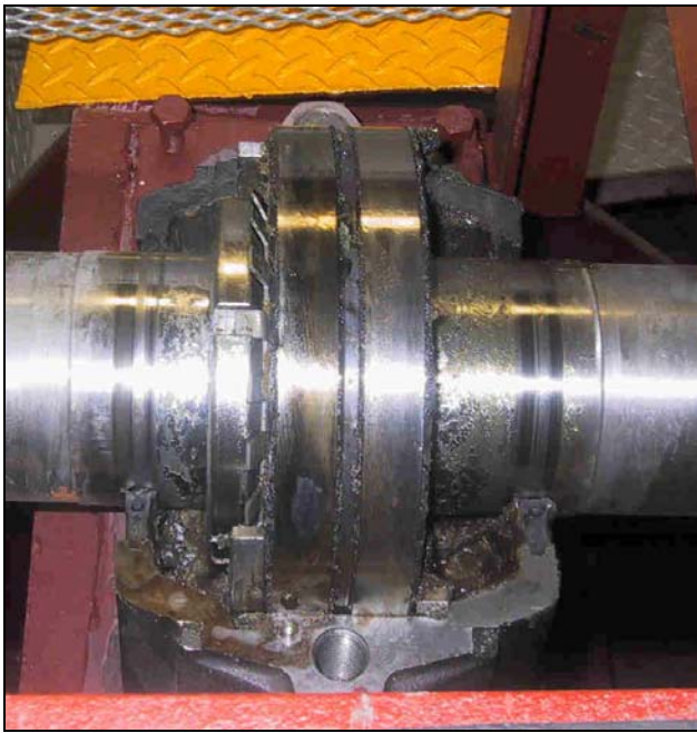
Photo 1 Lineshaft Bearing – Bearing Cap Removed (Note: Left side shows over-heating has occurred)
