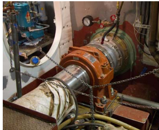
Photo 2 LCS 3 Port Boost Waterjet Lineshaft, Bearing and Seal
